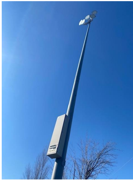
Softball Lighting Pole
